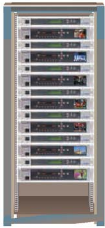
56 Channels headend, cable tv distribute.
